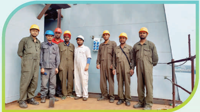
Installation of 45 Nos. of Industrial Electrical Extension Board on Yard 3022 on 14 Jan 23
