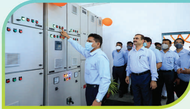
Inauguration of 480 KVAR APFC Panel at Building Berth Sub-station on 11 Apr 2022
