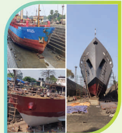
GRSE KPDD Unit set record by simultaneously repairing ICGS Vijaya, ITT Tiger & PV Ma Ganga at all three docks on 24 Mar 23
